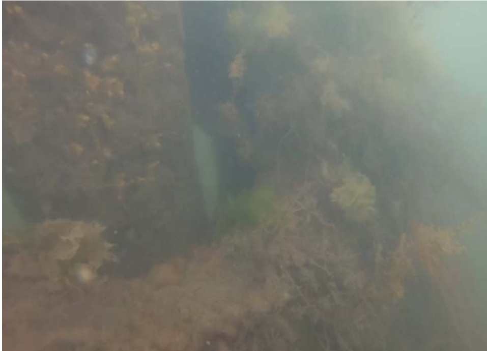
Photo 2: Submerged tire on Pile No. 4.
