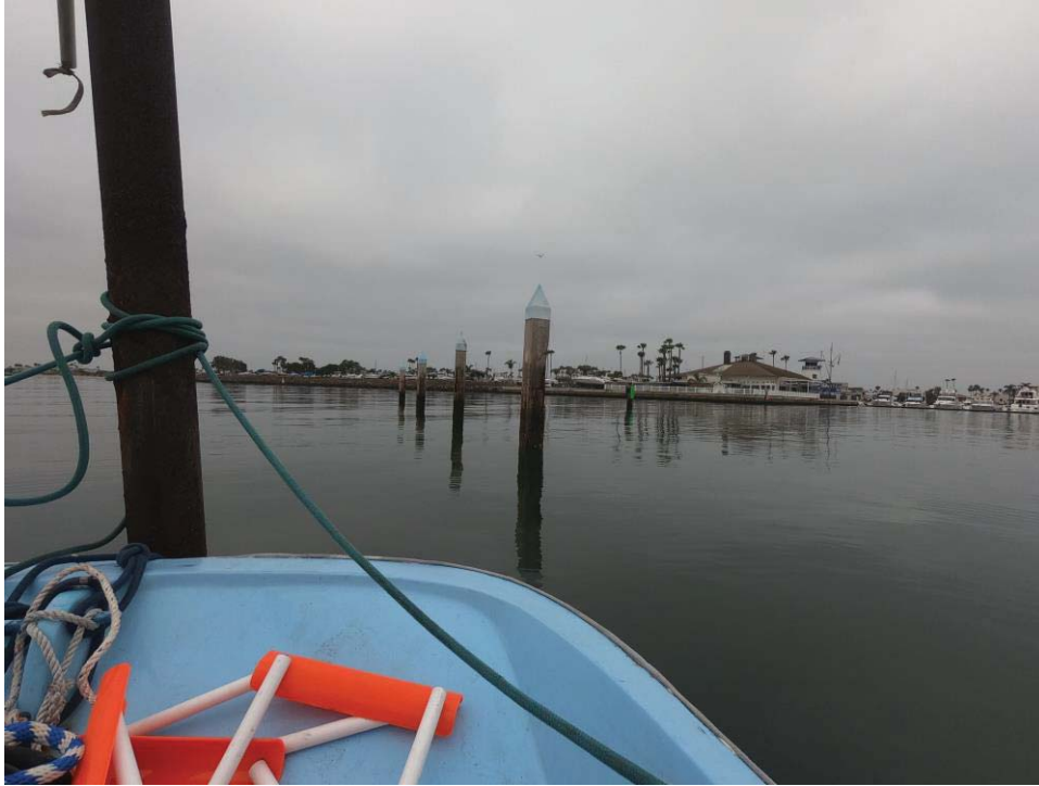
Photo 1: Dive skiff attached to a boat mast looking southwest at the southerly 4 piles that made up Tire Island. By zooming in, one can see the badly deteriorated condition of the concrete piles.
