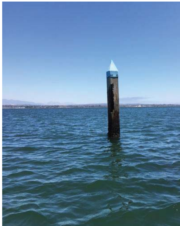
Photo 4: Close-up of badly deteriorated condition of Tire Island piles.
