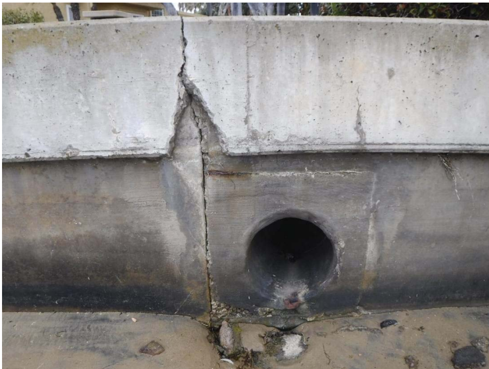
Photo 8: Mardi Gras North, Storm Drain between Lots 17 and 21. Pile cap above storm drain penetration has significant crack; concrete is broken and missing.
