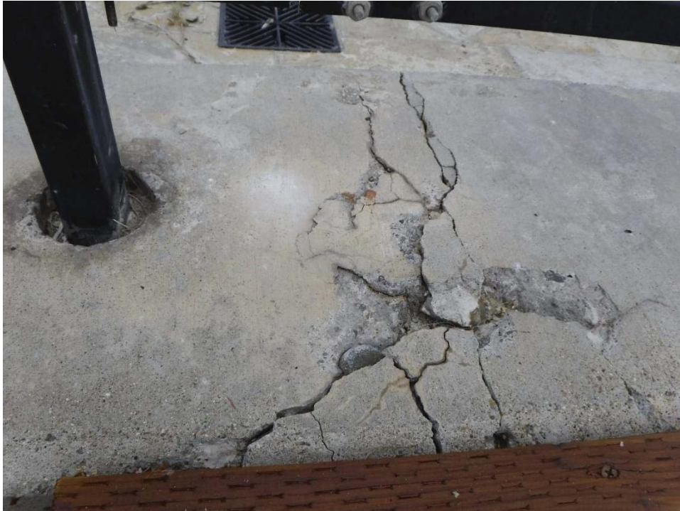
Photo 7: Mardi Gras North, Lot 23. Cracks in pile cap have approx.. 0.375 inch aperture; concrete is breaking apart.
