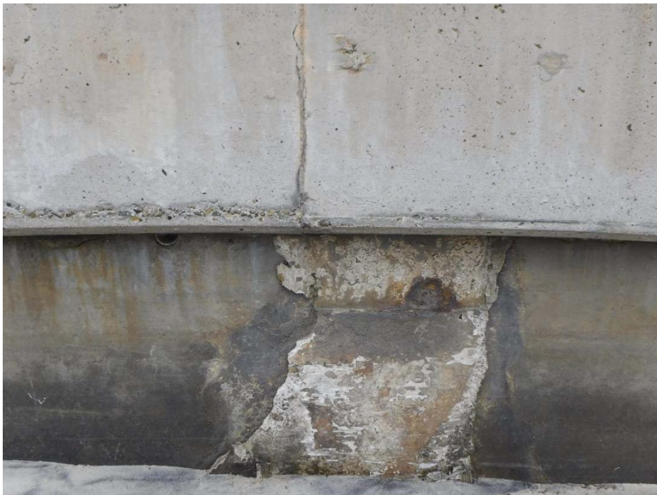
Photo 4: Mardi Gras South, Lot 35. Concrete spalling where bulkhead turns approximately 15 degrees.
