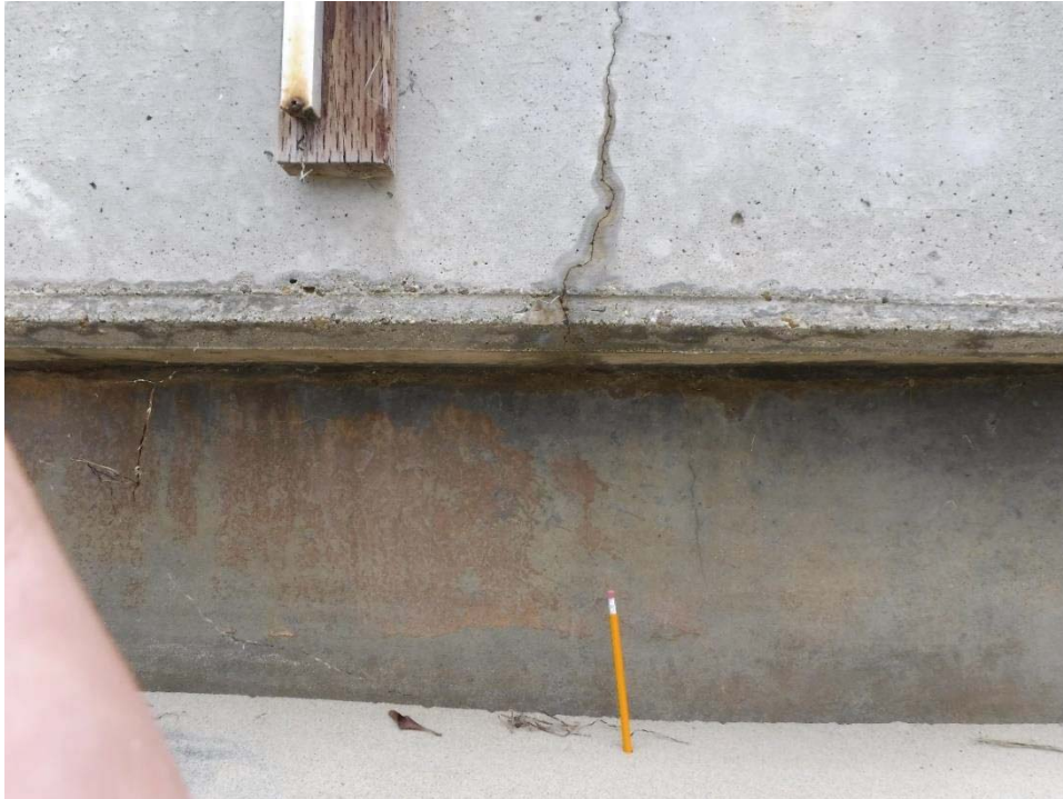
Photo 3: Mardi Gras South, Lot 37. Diagonal crack with light rust staining on panel cap.
