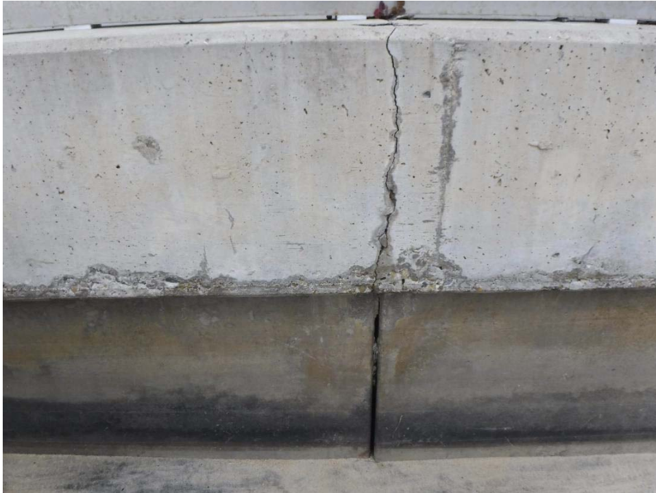
Photo 5: Mardi Gras North, Lot 27. North side of lot has significant crack and spalling.
