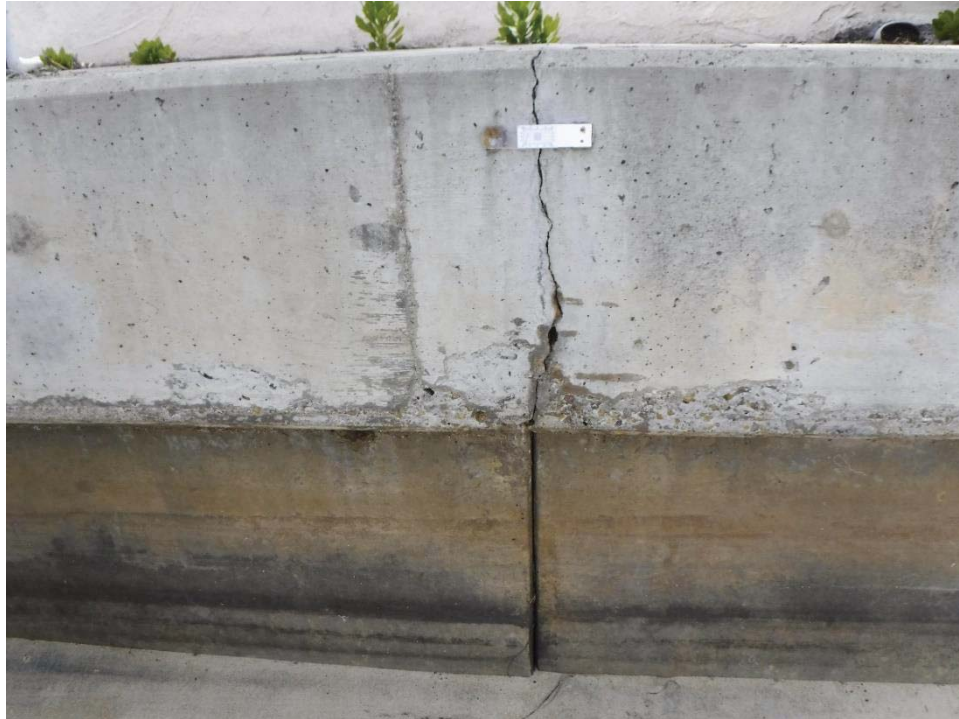
Photo 1: Mardi Gras South, Lot 67. Vertical cracks above panel joint.
