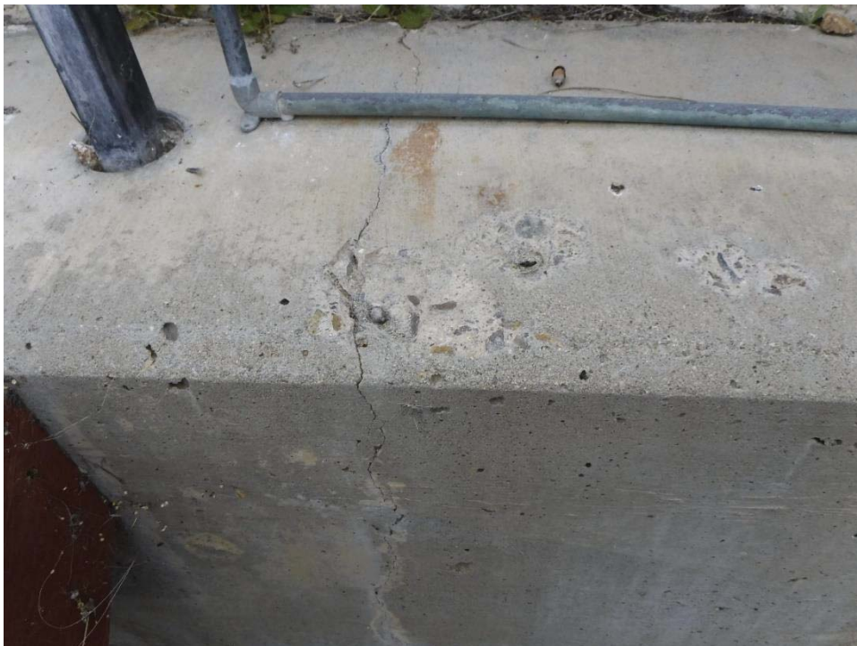
Photo 6: Mardi Gras North, Lot 25. Cracking in pile cap.
