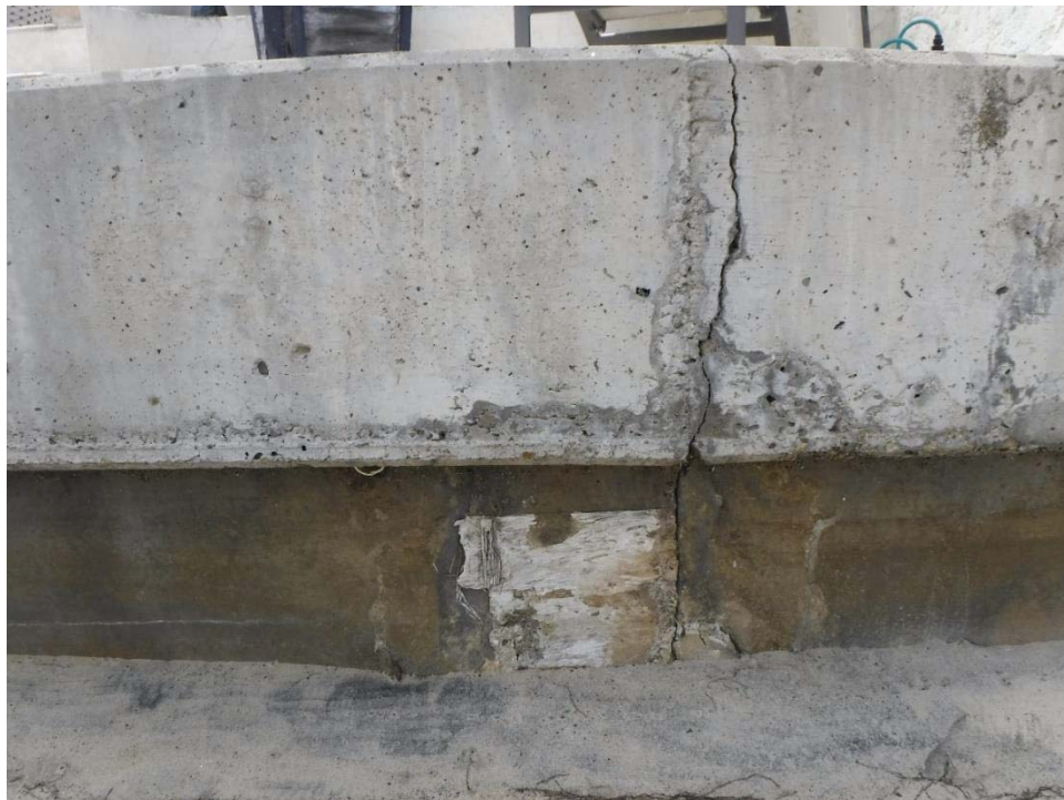
Photo 2: Mardi Gras South, Lot 59. Diagonal panel crack.
