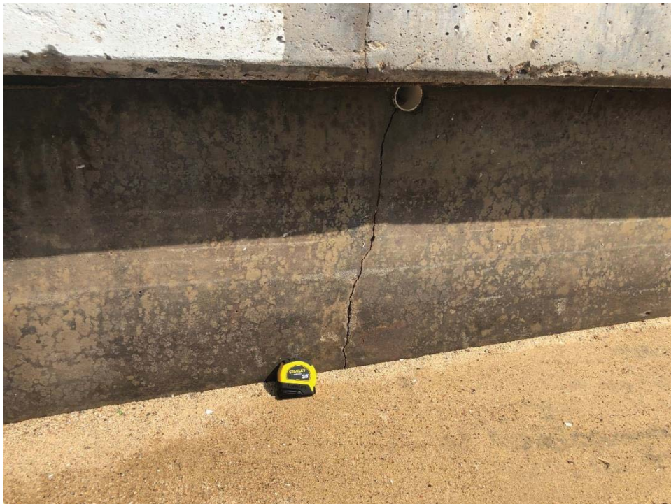
Photo 4: Port Royale Village between Lots 9 and 13. One vertical crack and two minor vertical cracks in panel.
