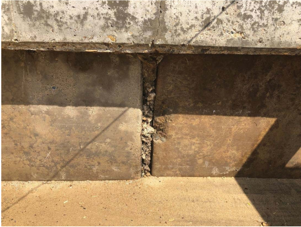
Photo 3: Port Royale Village, Lot 17. Northern panel joint offset and spalling, approx.. 2-inch aperture with deteriorating patch.
