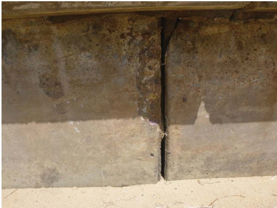
Photo 2: Port Royale Village, Lot 25. Significant crack above spalling panel joint.
