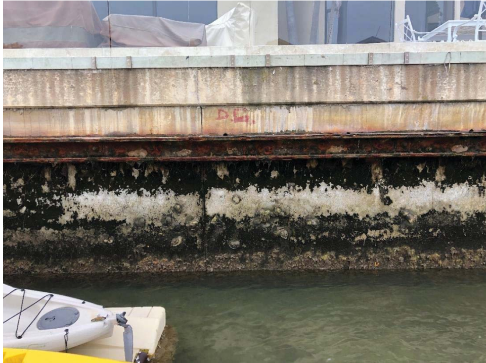
Photo 11: Spinnaker Way, north side of Lot 4. Steel whaler is badly corroded.
