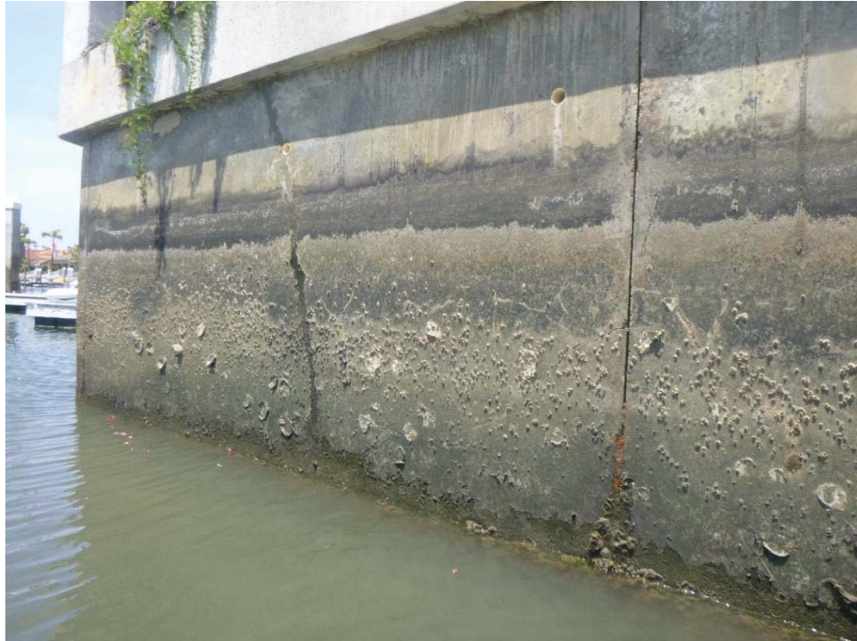
Photo 5: Blue Anchor Cay, Lot 4 southeast corner. Minor spalling, west side of corner panel.
