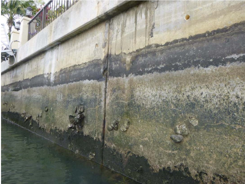
Photo 1: Blue Anchor Cay, Lot 36, Panel 3. Horizontal cracks, spalling between Lots 36 and 34.
