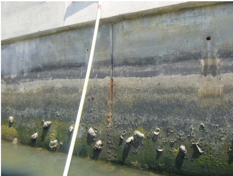
Photo 4: Blue Anchor Cay, Lot 8 Panel 1. Rust at joint.
