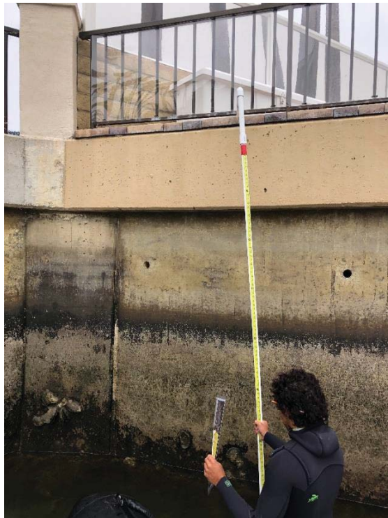
Photo 8: Spinnaker Way, second panel east of Lot 4/6 P/L. Vertical crack and spall.
