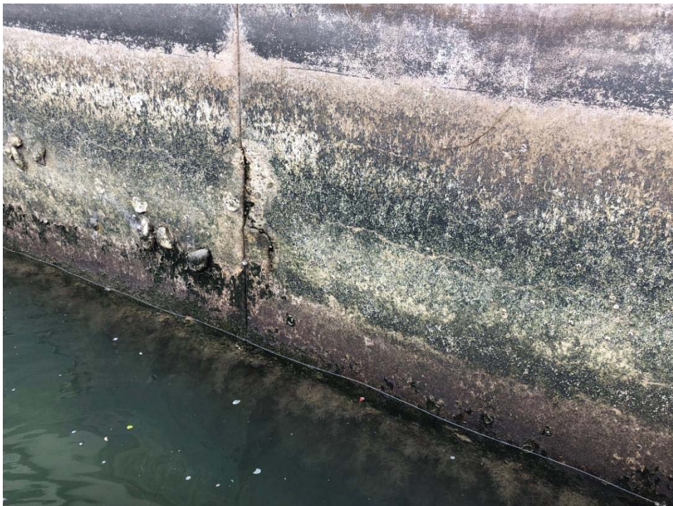
Photo 2: Blue Anchor Cay, Lot 30, west edge of west panel. Cracking and spalling.
