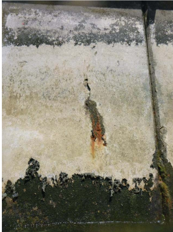
Photo 1: Port of Spain, One Panel North of Lot 77 Gangway. Rust and major cracking.
