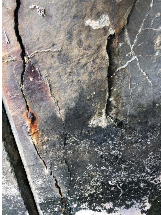
Photo 5: Port of Spain, Lot 3. Panels are badly cracked.
