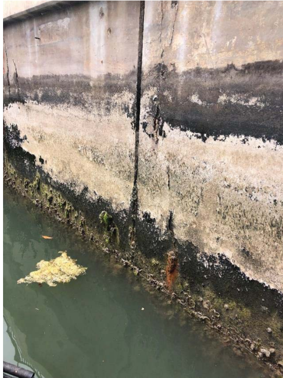
Photo 7: Port of Spain, Lot 3. Panels are badly cracked.
