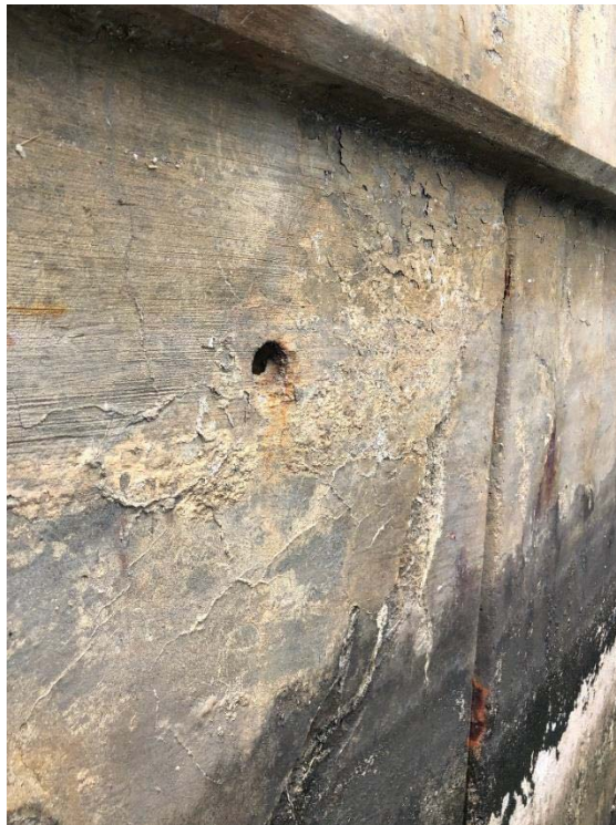
Photo 2: Port of Spain, 12 Panels north of Lot 53 Gangway. Spalling at panel joint.
