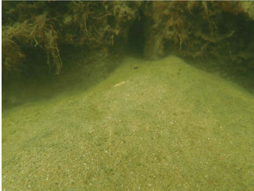
Photo 3: Port of Spain, 7 th Panel North of Lot 29/31 Property Line. 1-inch joint with 6" w x 3" h talus pile.
