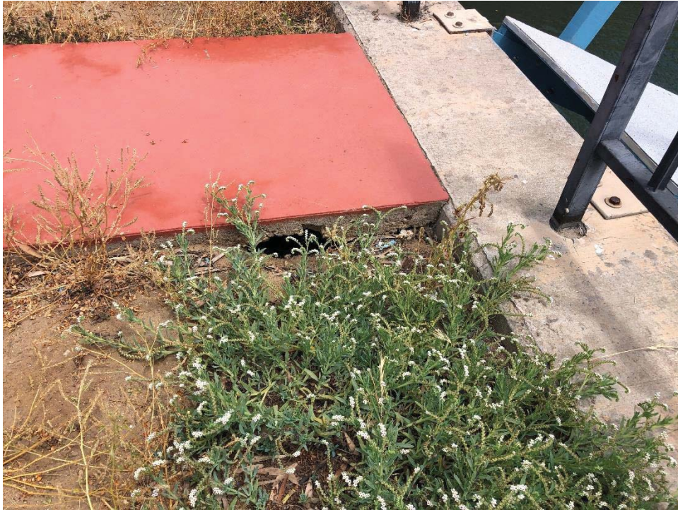
Photo 11: Port of Spain, Lot 3. Void under walkway suggests some lost ground.
