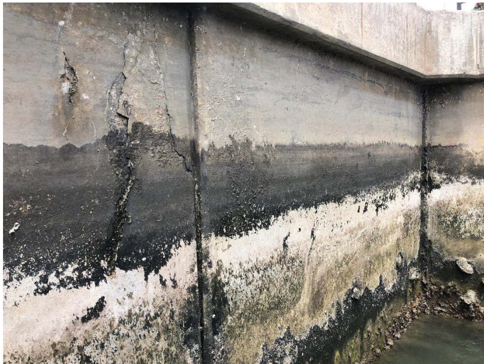
Photo 10: Port of Spain, Lot 3. Panels are badly cracked.
