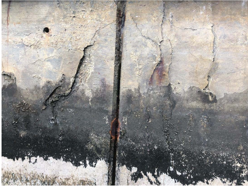
Photo 9: Port of Spain, Lot 3. Panels are badly cracked.
