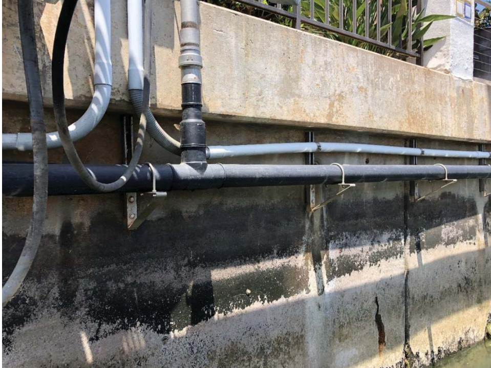
Photo 14: Port of Spain. This bulkhead has unusual utilities attached right under the pile cap.
