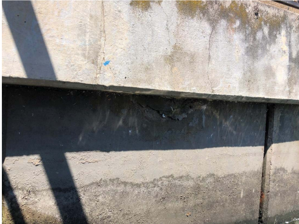
Photo 13: Catspaw Cape. Delamination and cracks, spalling under pile cap.
