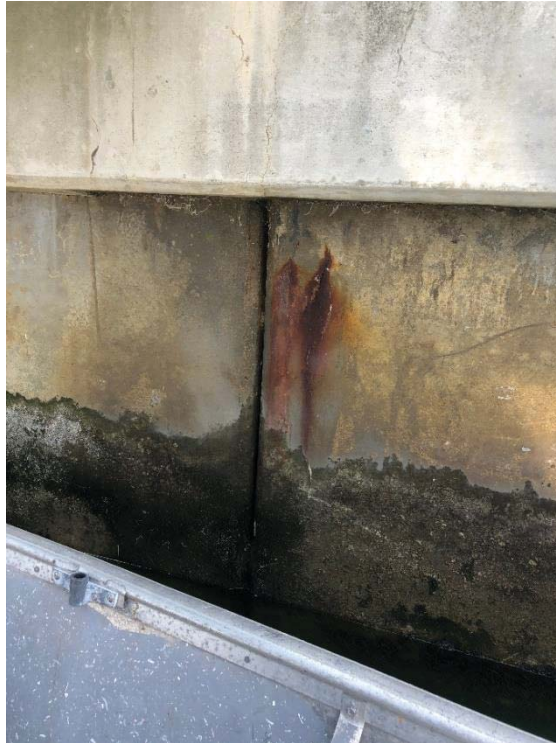
Photo 5: Catspaw Cape, Lot 49. Crack with rust stains right of joint.
