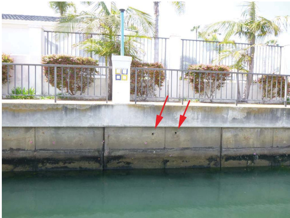
Photo 7: Note two bulkhead penetrations below area where voids were detected.
