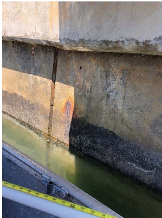
Photo 10: Catspaw Cape, Gangway between Lots 13 and 15. Rust and minor vertical cracking.
