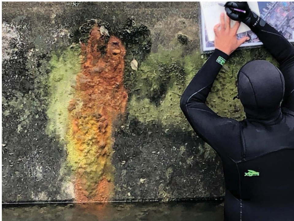
Photo 2: Catspaw Cape, first panel south of Lot 63 gangway. Badly rust bleeding.
