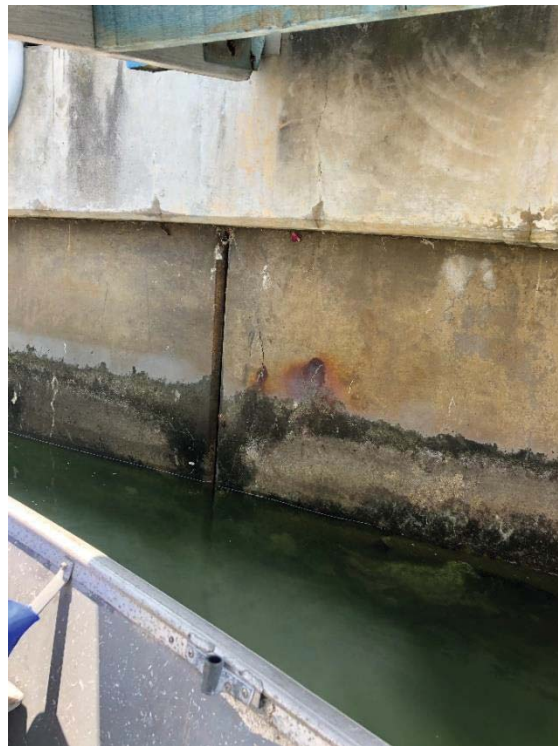
Photo 8: Catspaw Cape, CCHOA west of gangway. Under gangway, vertical crack and rust.
