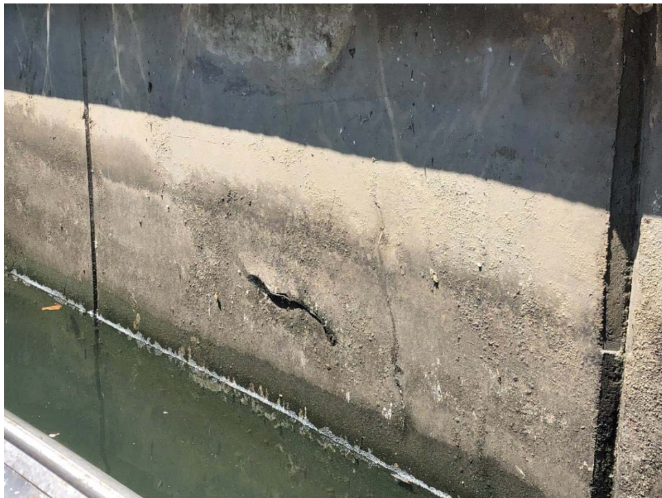
Photo 14: Catspaw Cape, Lot 1, north of gangway. Cracking and spalling.
