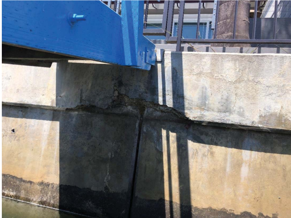
Photo 11: Catspaw Cape, Lot 13 gangway. Pile cap broken off, spalling; 1-inch opening at joint, no talus.
