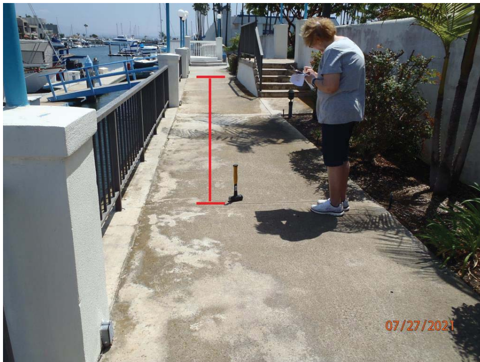
Photo 6: Voids detected under sidewalk from east side of stairs to approx.. 20 feet west of stairs. Also randomly detected voids adjacent to the bulkhead in other locations along the north bulkhead.
