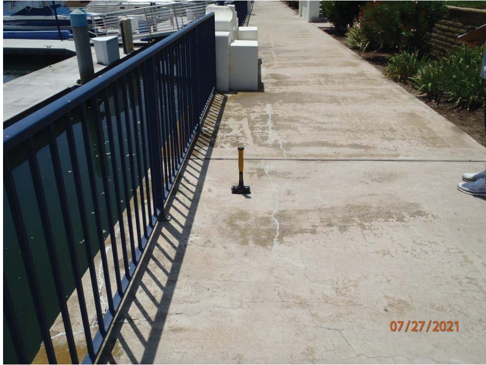
Photo 1 – Sidewalk at southeast corner of Jamaica Village midway between Half Moon Bend and Ginger Tree Lane shows evidence of settlement and voids.
