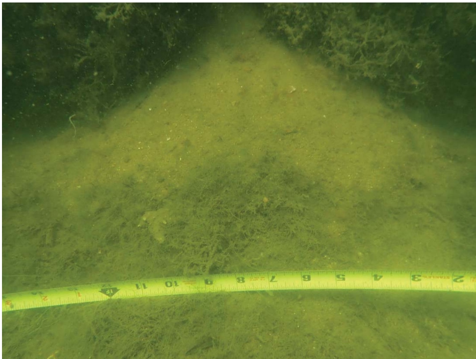
Photo 6: Kingston Court S, talus pile (12" w x 6" h) at 1-inch-wide joint west of Gangway 11.
