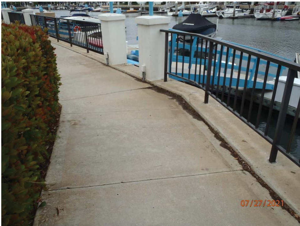
Photo 12: Note numerous sections of sidewalks show evidence of settlement adjacent to the bulkheads. Gangway 20 in background.
