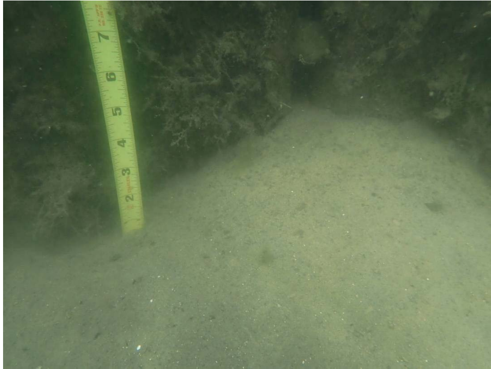
Photo 3: Kingston Court E, talus pile (9" w x 3" h) at 1-inch-wide joint south of Gangway 4.
