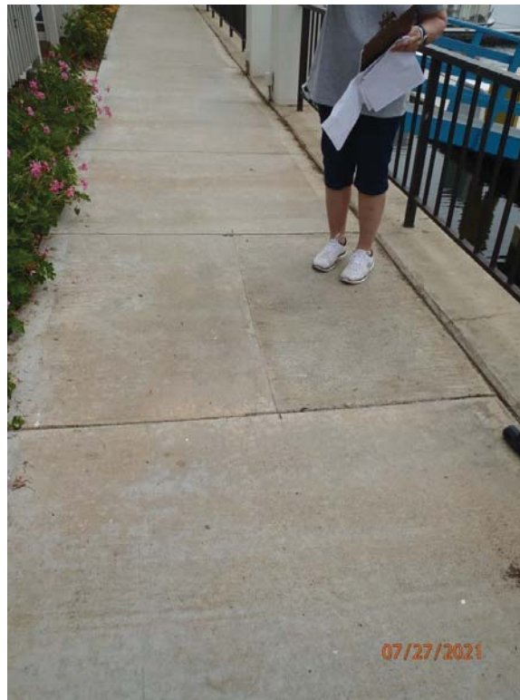
Photo 8: West of Gangway 16. Void detected under concrete patch in sidewalk on southerly end of Kingston Court.
