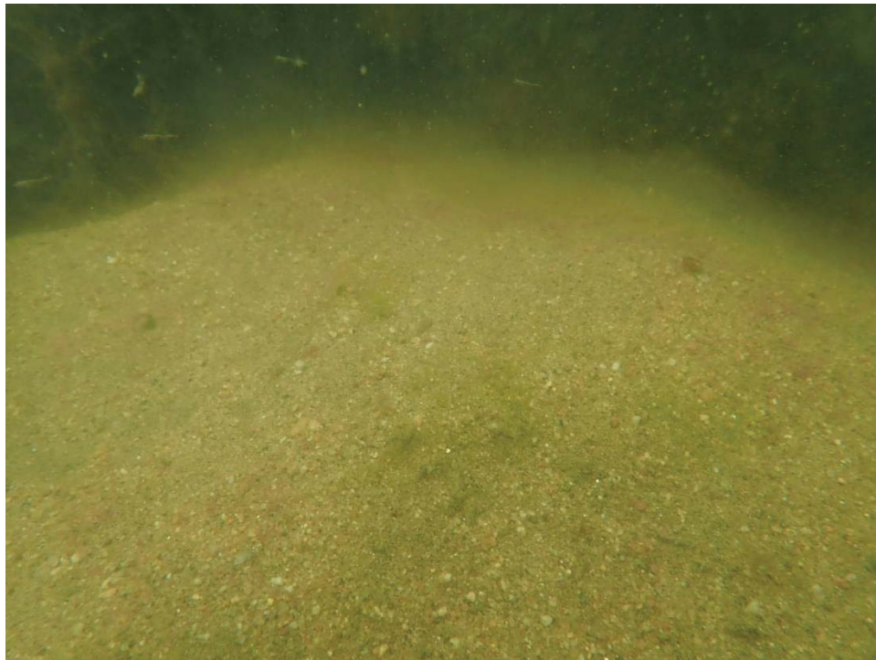
Photo 10: Kingston Court W. Small talus pile at 1.25-inch-wide joint 85 feet south of Gangway 17.
