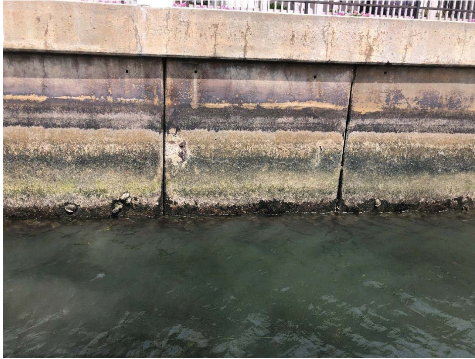
Photo 7: Kingston Court, fifth panel from west end (southern corner). Significant cracking.
