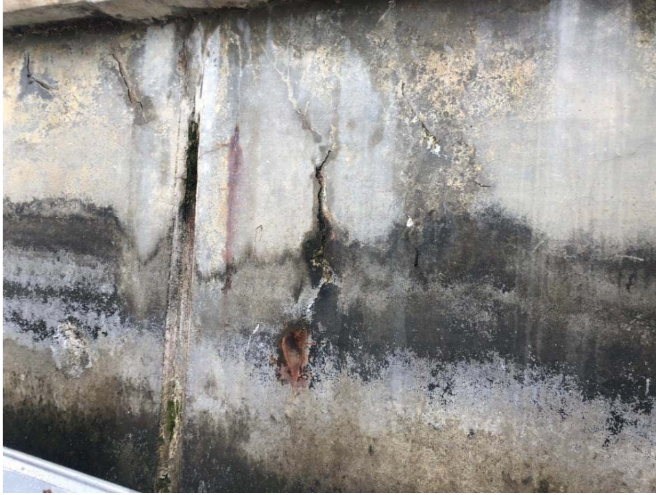
Photo 1: Kingston Court, Lots 3-13, 32 feet south of northern corner. Vertical crack bleeding rust.
