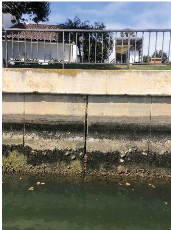
Photo 4: Kingston Court S (end of east cul-de-sac), panel under second gangway. Soil on top of grout (grout breach).
