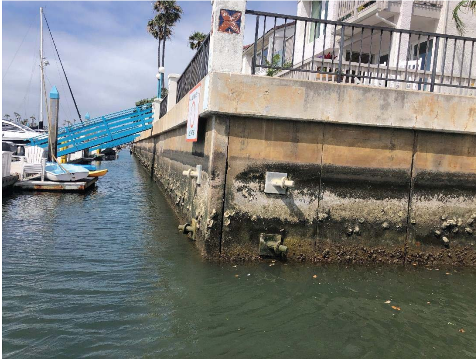
Photo 5: Kingston Court, panel under second gangway. Two diagonal tie rods have been installed.
