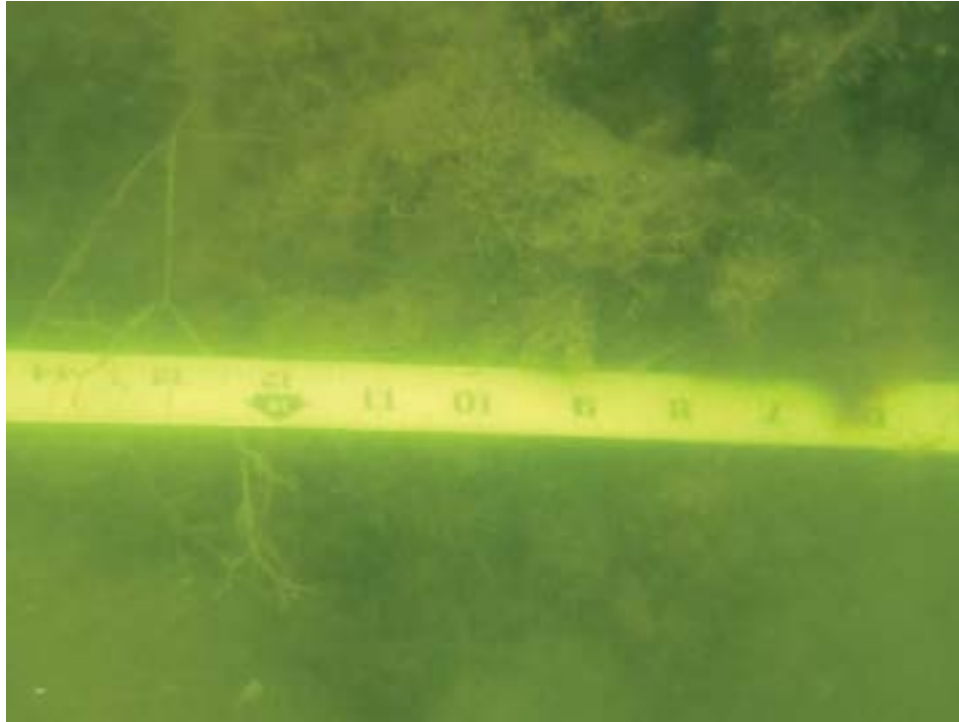
Photo 3: Antigua Court. Talus pile just south of Gangway 4. Although not visible in photo, joint width is 1 inch.
