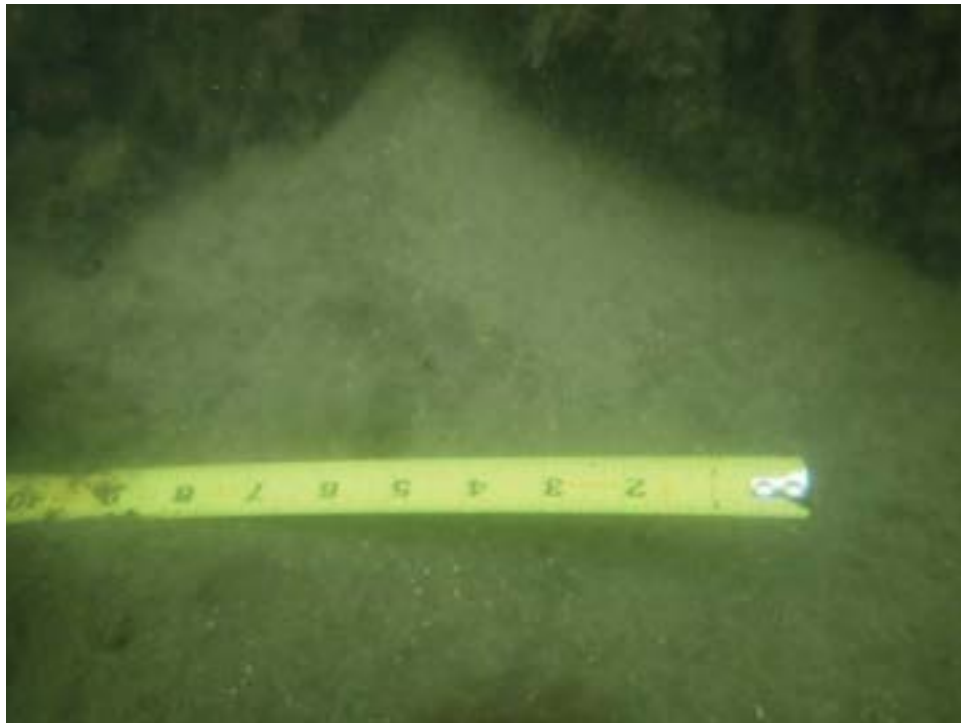
Photo 6: Antigua Court. 6-inch-high talus pile at northwest corner joint
