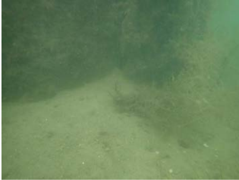
Photo 7: Antigua Court. 6-inch-high talus pile at northwest corner joint
