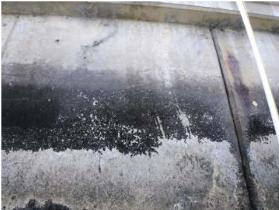
Photo 18: Antigua Court, Lot 3/5 P/L, north side of gangway. Panel joint widens to >2.5 inches at top of panel and tapers to >0.25 inch at waterline. Minor horizontal cracking approximately 2 to 3 feet below pile cap.
