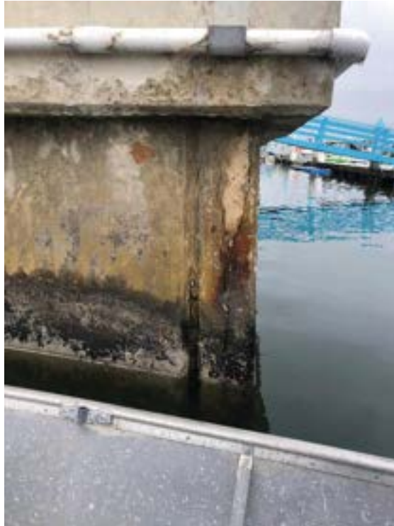
Photo 13: Antigua Court, northeast corner (north wall). Vertical cracks, rust, spalling, wide joint, talus observed.
