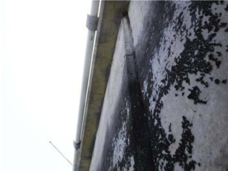
Photo 17: Antigua Court, Lot 5, 5 feet south of P/L. Panel joint is rotated approximately 0.75 inch at the top.
