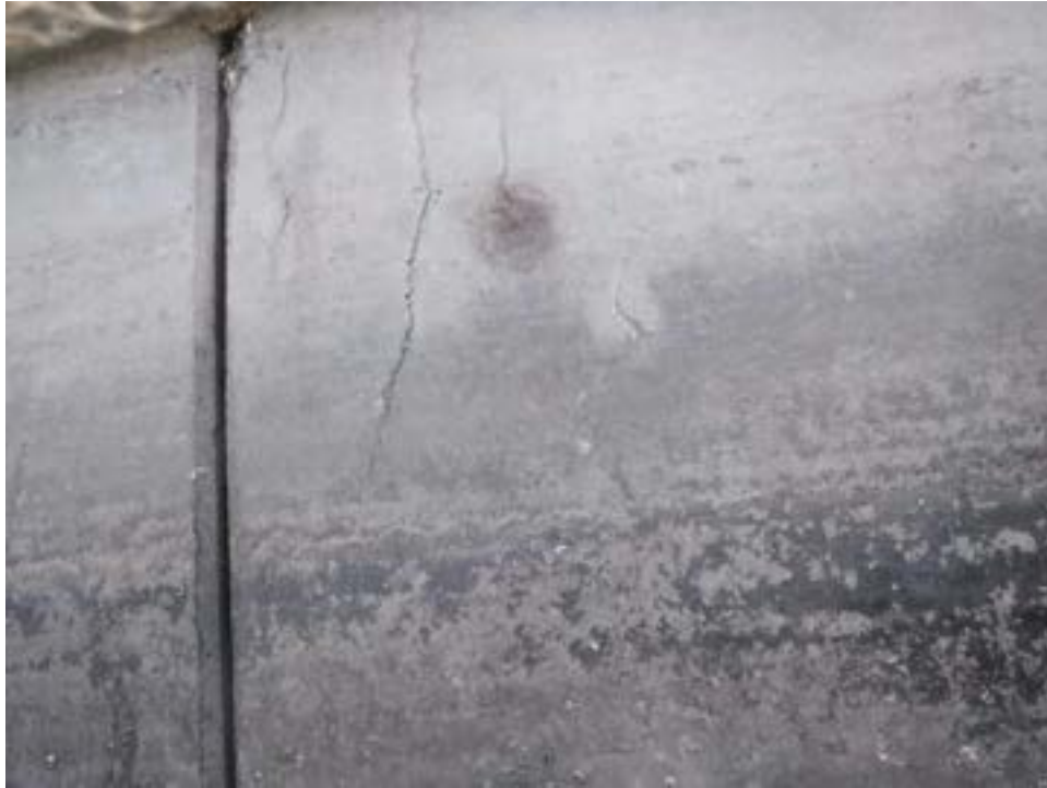
Photo 19: Antigua Court at Grand Caribe causeway. Vertical cracking, minor spalling on bulkhead panel.
