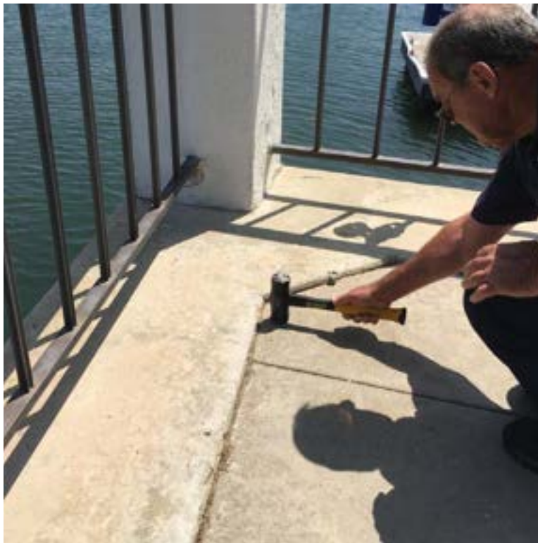
Photo 12: Antigua Court. Checking for voids under sidewalk at common area, northeast corner of Antigua Court.
