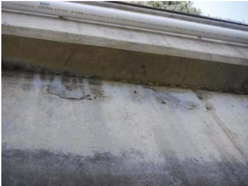
Photo 16: Antigua Court, Lot 11, 5 feet south of P/L. Spalling under pile cap.
