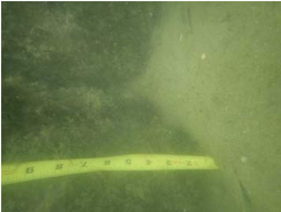
Photo 2: Antigua Court. Talus pile just south of Gangway 2 (joint approx.. 10 feet southerly of gangway).
