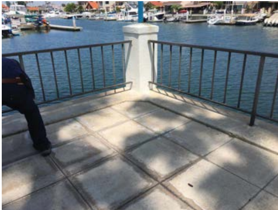
Photo 4: Antigua Court. Checking for voids under sidewalk at common area, northwest corner of Antigua Court.
