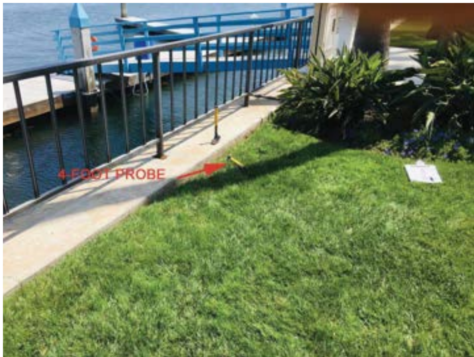
Photo 10: Antigua Court. Note grass area experiencing settlement. Also note handle of 4 foot probe, indicating loose soil behind bulkhead.
