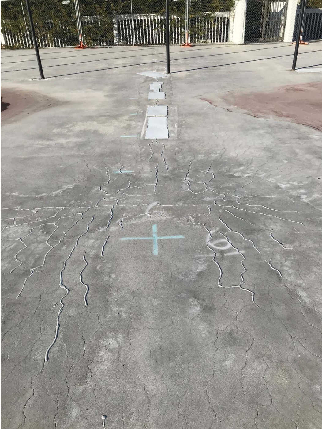
2022 0124 Photo 003 Support Column Radial Cracking
