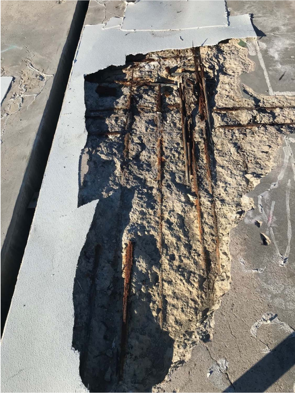
2022 0124 Photo 001 Disintegrated Cables Center Line
